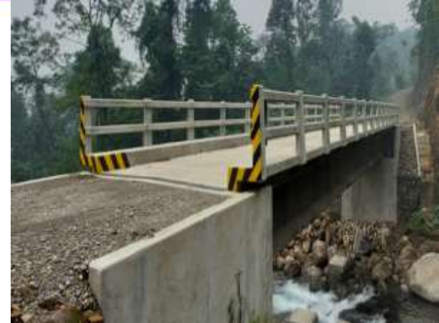
Const. Puente Vehicular Roberto Padilla-Central Jatun Pampa D.10 Villa Tunari (CONVENIO FDI)
